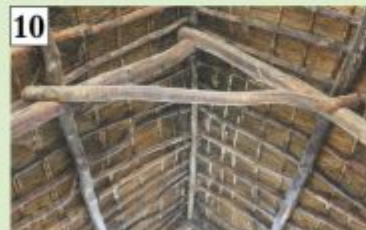
The slave house still has a very old thatched roof with reeds from the original reed bush.
